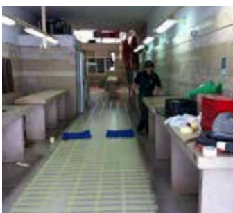
Tiled floor before
